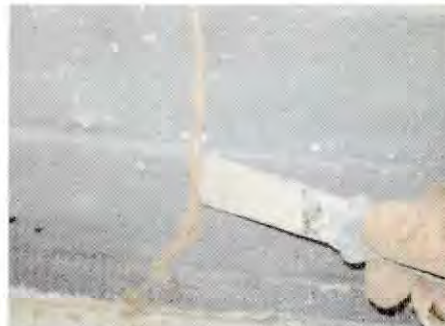
Mud tubes on concrete siding
