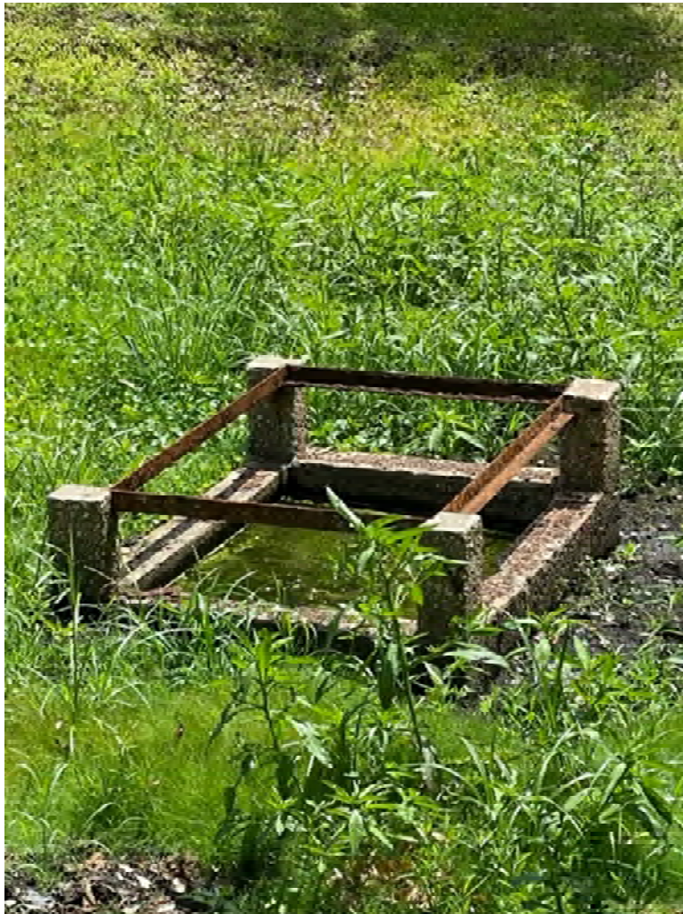
Photo 1 – Missing grate (S10) located in the sump on the north side of Cardinalwood at the curve.
